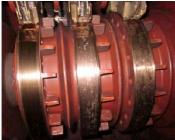
Figure 1. A rotor with damage detected by the QuickServer service report.
